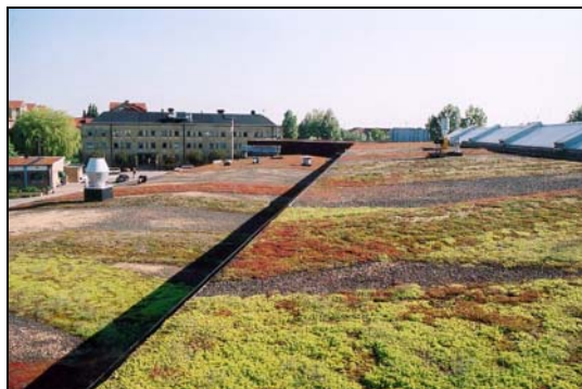
Figura 08. gustenborg (Scandinavia Green Roof Inst.)
